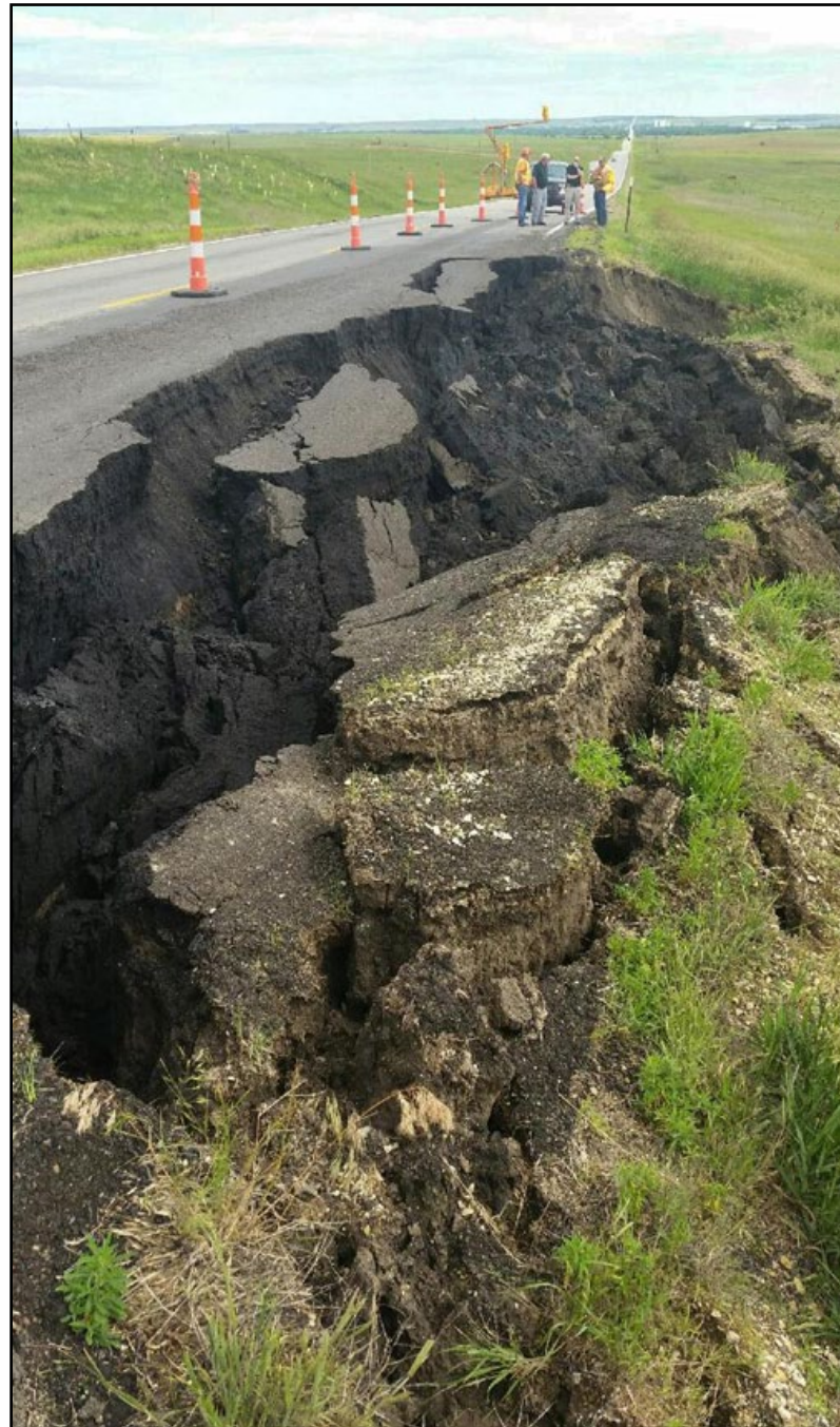
Two weeks after the first slope failure due to heavy rains in May, a second slope failure took place on U.S. 281 south of Osborne about 100 yards from the first failure. The Osborne, Smith Center and Stockton Subareas, the Phillipsburg Area and District bridge crew are working on the repairs.
