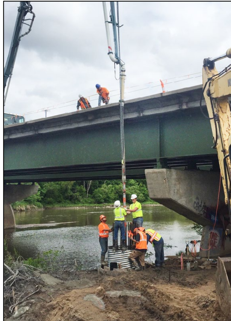
Work continues on the Arkansas River Bridge in Wichita as crews pour drill shafts.
