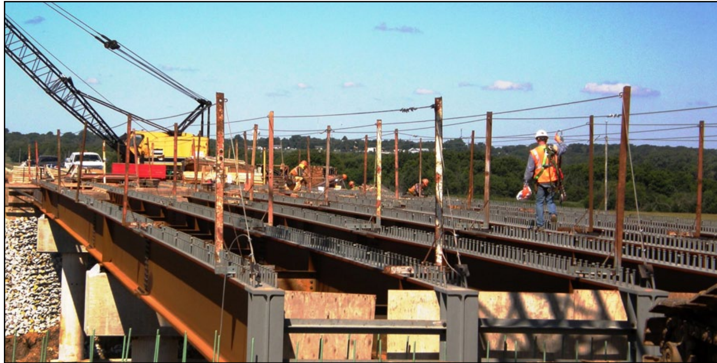
Work continues on the new U.S. 54 railroad overpass east of Yates Center. Crews with A.M. Cohron & Son, Inc., of Atlantic, Iowa, work on bridge deck components prior to the August concrete deck pour. Traffic is continuing to detour around the project by way of U.S. 169, K-39 and U.S. 75. The $4.1 million project will be completed this autumn. Chris Meyer's bridge squad and Aaron Frits' road squad designed the project.
