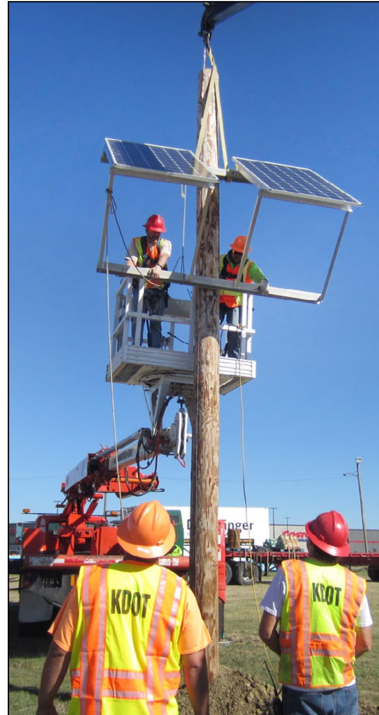
The Wichita Area Crew installed solar panels last week for a video camera that will monitor work zone traffic on the freeway project at U.S. 54 and Webb Road. Live images will be viewed in the WICHway Traffic Management Center, and KTA staff is working to provide the video to the public via the project website.
