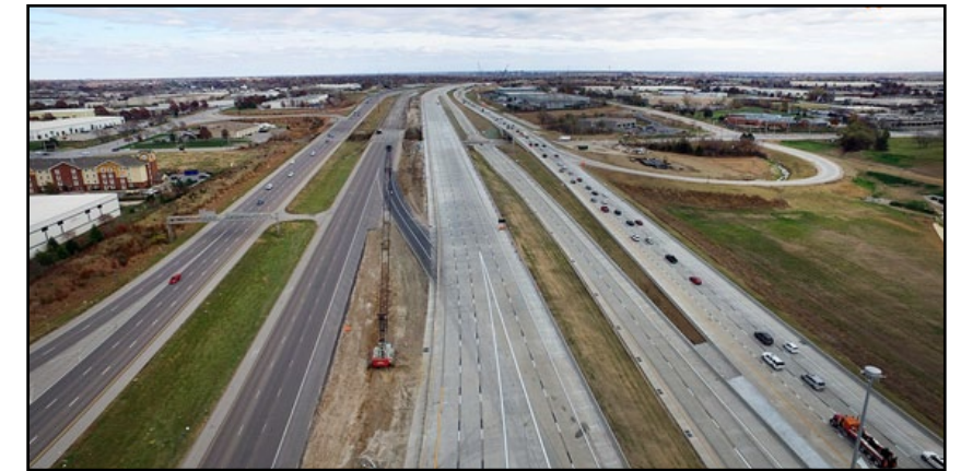
This view of eastbound I-435 at Lackman Road shows the roadway before traffic was switched over on Sunday night to the newly-constructed pavement for the winter.
