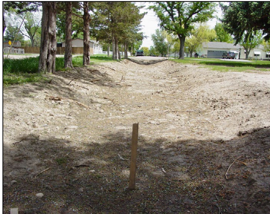
A drainage ditch was built to reduce runoff problems once upgrades to the Syracuse Subarea are complete.
