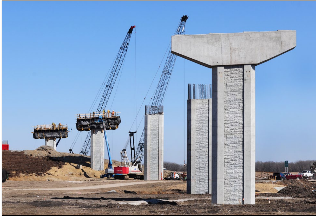
Construction is taking place on the pier columns for the bridge that will carry traffic from eastbound K-10 to westbound 23rd Street near existing K-10 in Douglas County. There are a total of 26 bridges on the South Lawrence Trafficway project that is underway.
