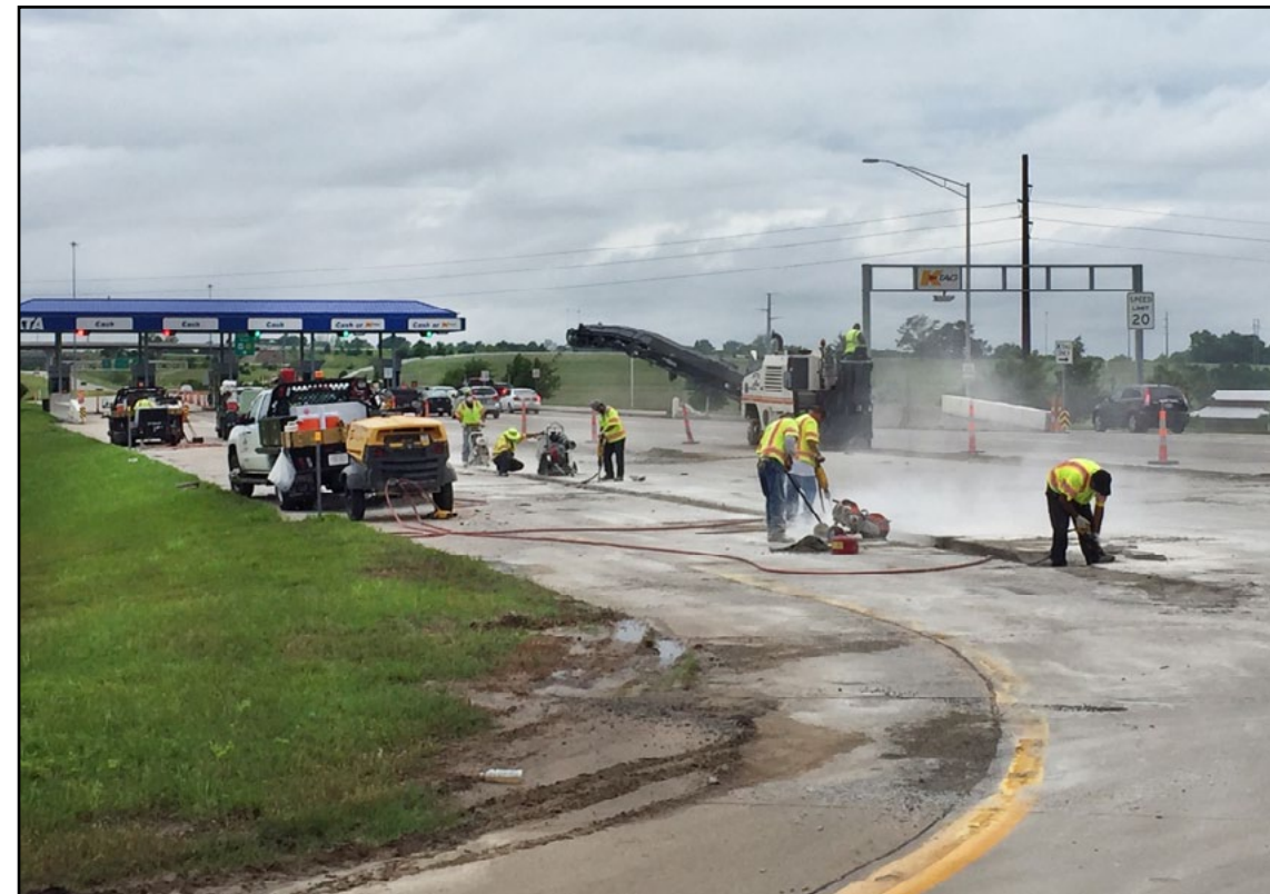
A concrete pavement patching project at the Kansas Turnpike's two east Topeka toll plazas (mile marker 182 on I-470/KTA and mile marker 183 on I-70/KTA) continues. It also includes four connecting ramps to K-4 and I-70. The repairs at I-470/KTA are near completion. The repairs at I-70/KTA are expected to be completed mid-June. Until then, travelers can experience periodic lane closures and possible width restrictions.
