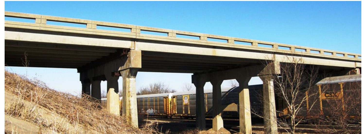
KDOT will start a project in March to demolish and replace the Union Pacific Railroad overpass on U.S. 54 just east of Yates Center. The existing overpass was built in 1936 and modified in 1970. Traffic will be detoured on U.S. 75, K-39 and U.S. 169. A.M. Cohron & Son of Atlantic, Iowa, is the contractor of the $4.2 million project that should be completed this fall. Aaron Frit’s road squad and Chris Meyer’s bridge squad designed the project.
