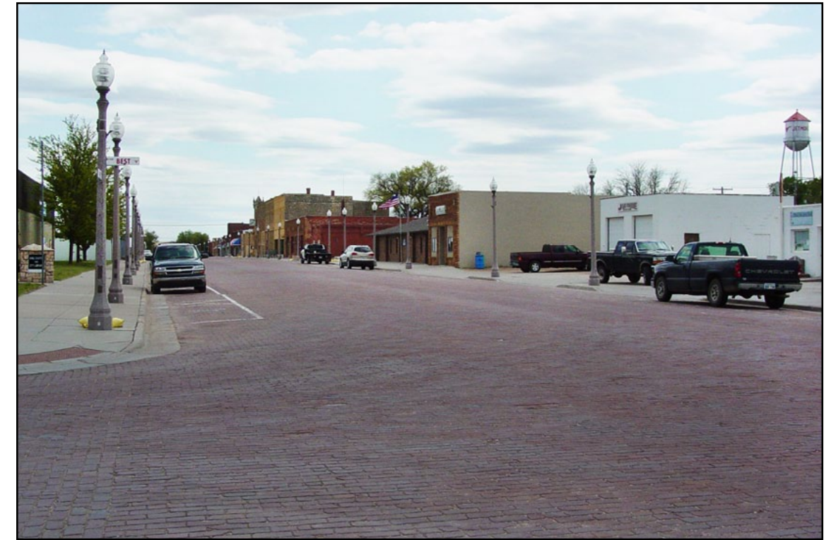
A geometric improvement project on Main Street (U.S. 283) in Jetmore is ready to start this week. The project will replace a two-block stretch of brick pavement with concrete pavement, from Highway Street to Best Street. The contractor is J-A-G Construction Company of Dodge City at a cost of $939,000, with KDOT's contribution capped at $700,000. The work is expected to be completed by August.
