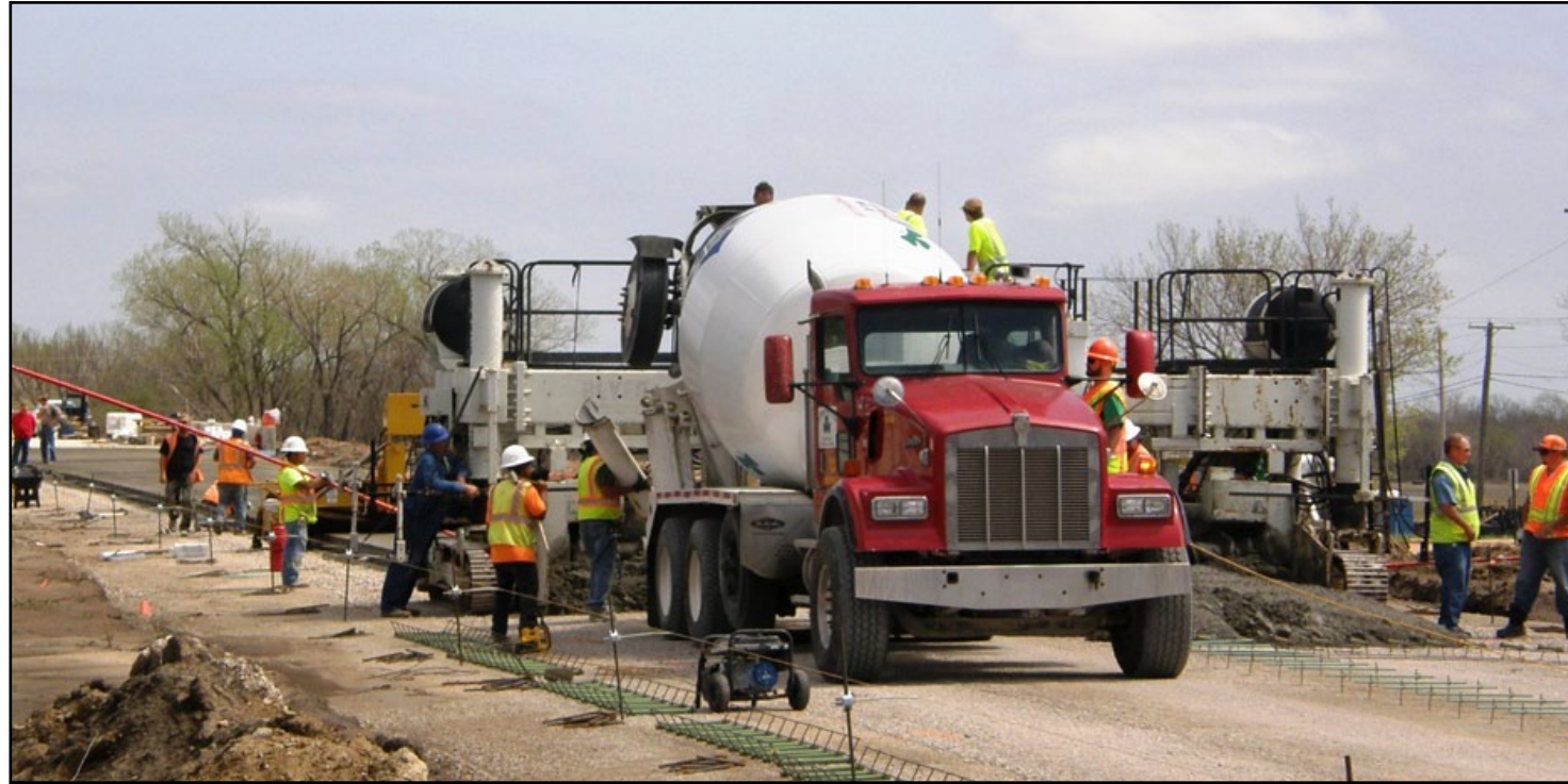
The new K-39 bridge at the east edge of Chanute is nearing completion. Crews with project contractor B&B Bridge place the concrete for the bridge approach on the west side. The $1.7 million project should be finished this summer.
