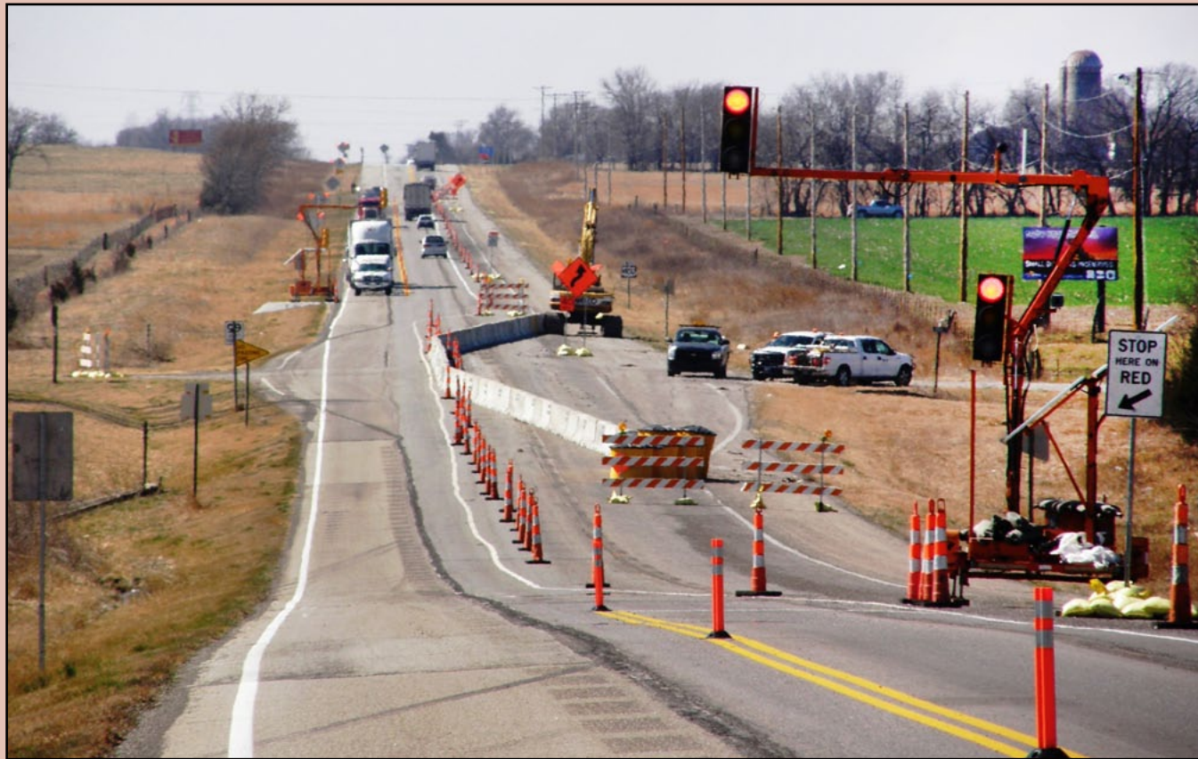
East of Parsons, a $3.9 million project to add passing lanes on both sides of U.S. 400 and resurface the driving lanes began in early March. Temporary traffic signals have been activated at the location of a culvert replacement on the project. Shilling Construction of Manhattan is the contractor on the expansion, which should be completed by late summer. Steve King's road squad and Chris Meyer's bridge squad designed the projects.
