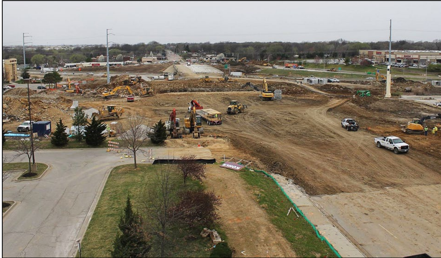
A view from the project webcam shows construction on the 95th Street/I-35 Diverging Diamond Interchange. Webcam photos and other information about the project can be found at http://jocogateway.com/ .
