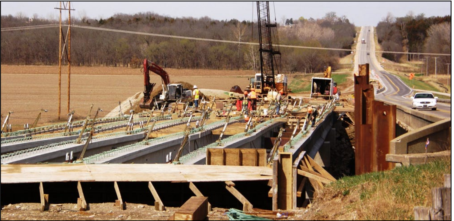
The deck of the new bridge over Pottawatomie Creek takes shape on U.S. 59 north of Garnett. Traffic is being carried on the existing bridge, at left. B&B Bridge Company of St. Paul is contractor on the $5.5 million project. Steve Rocker's road squad and Brad Rognlie's bridge squad designed the projects.
