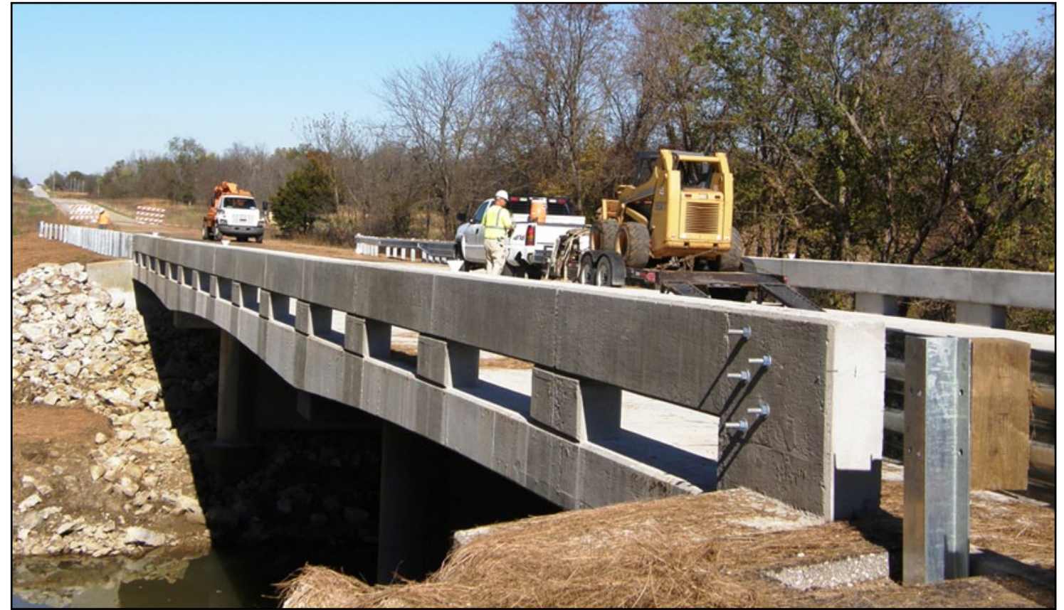
Finishing touches are applied to the Hinton Creek Bridge on K-3 before the new bridge opens to traffic. Located approximately three miles north of the west K-3/K-39 junction in Bourbon County, the bridge had been closed for replacement since March. King Construction Company, Inc., of Hesston was contractor on the $820,000 bridge project. Steve Rocker's road squad and Chris Meyer's bridge squad designed the projects.
