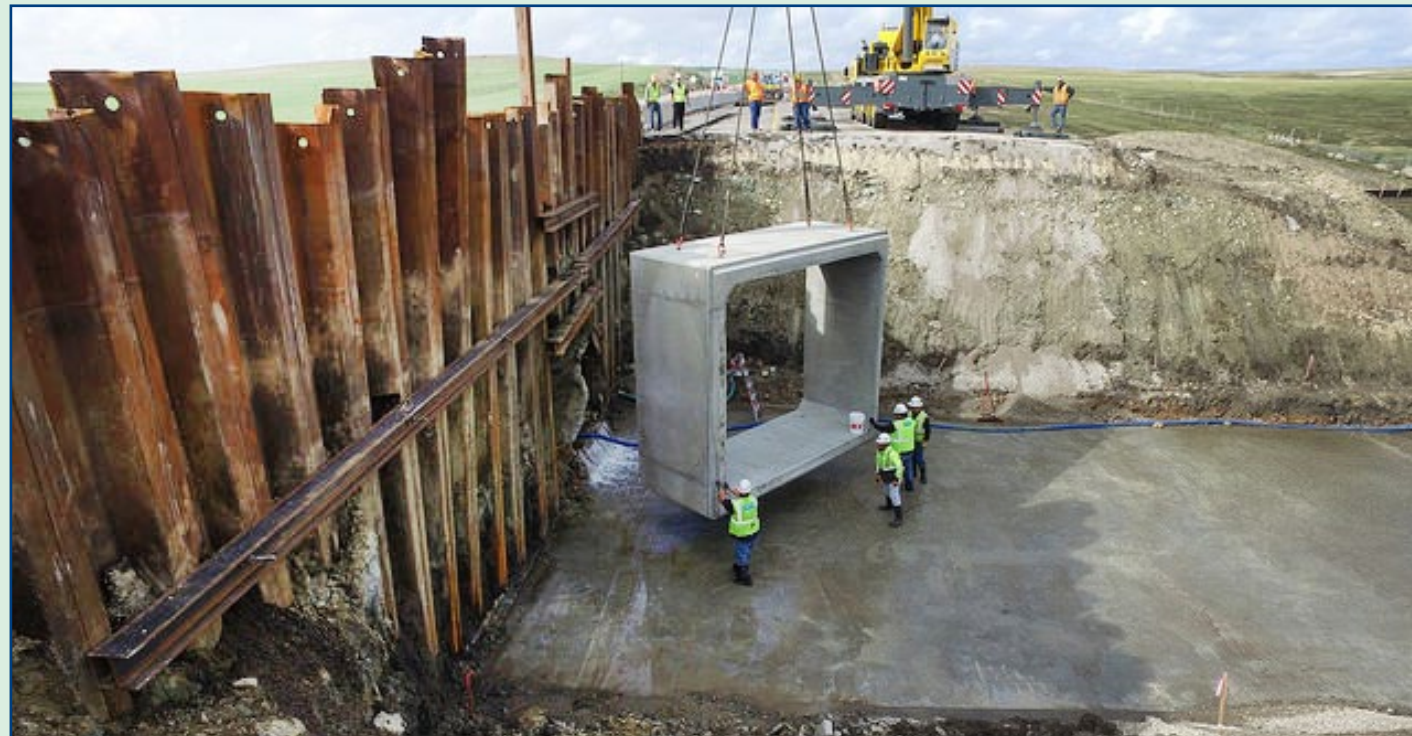
New box culverts were installed at mile marker 116 along the Kansas Turnpike this summer.
