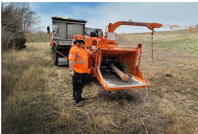
Equipment Operator Senior Gary Werth monitors a chipper used to turn trimmed trees into mulch during trimming along U.S. 54 west of Garden Plain. Photo by Ryan Wallace
