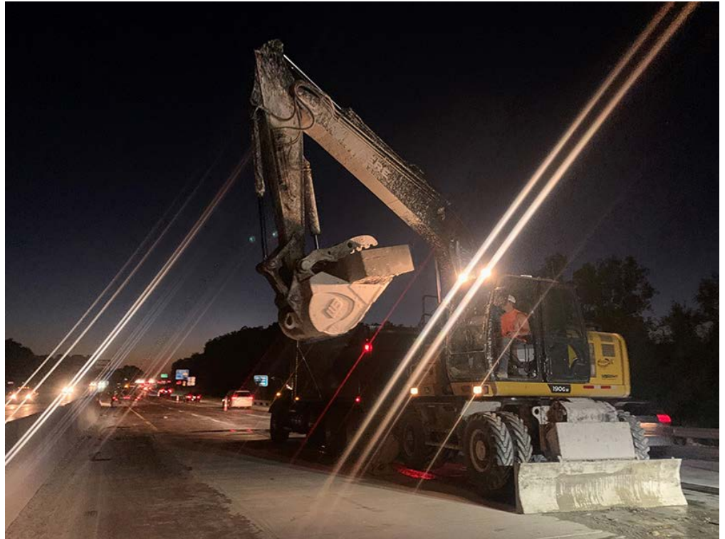
On westbound I-70, lane and ramp closures were scheduled overnight to limit interruptions to high-volume traffic. Photos by Delaney Tholen, District One
