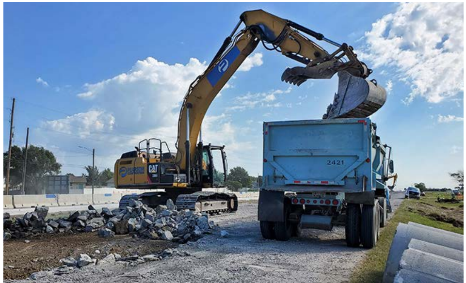
Crews work on road demolition preparing for the new RCUT intersection in Goddard on U.S. 54. Photo by Tracy Statton, District Five
