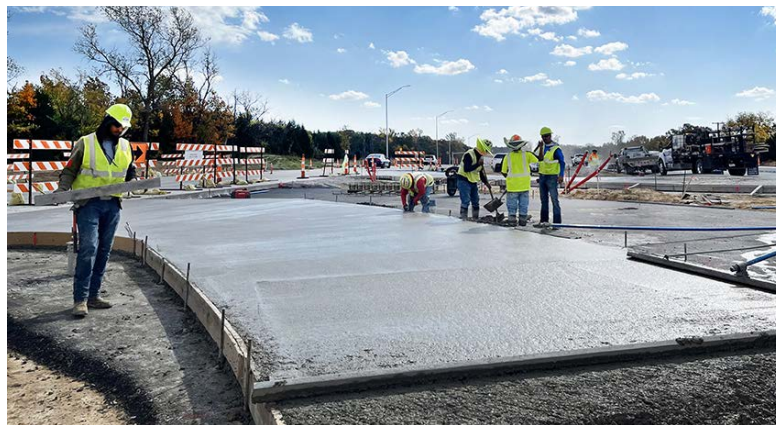
Crews building forms at the eastbound K-10/Kill Creek bridge deck replacement project worksite.
