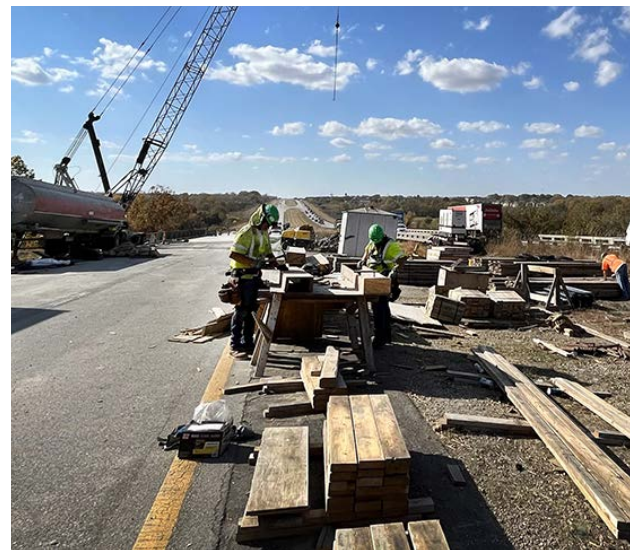
With traffic traveling head-to-head on the newly built northbound K-7 lanes at Parallel Parkway, new southbound K-7 lanes and RCUT turning lanes are in progress.
