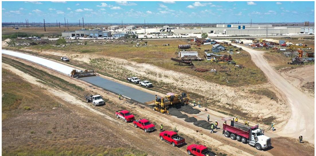
Crews from Wildcat construction pour concrete on 230th Avenue. The route is part of the Northwest Business Corridor located northwest of Hays. Photo by Driggs Design Group
