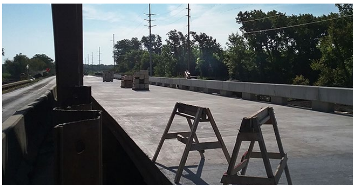
Each bridge is being replaced one half at a time. Signals control traffic. Photo by Priscilla Petersen, District Four
