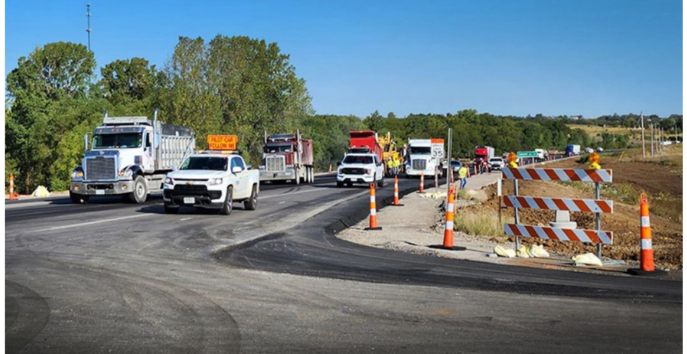
A pilot car leads traffic on U.S. 75 through the project's northern portion. Photos by Kate Craft, District One
