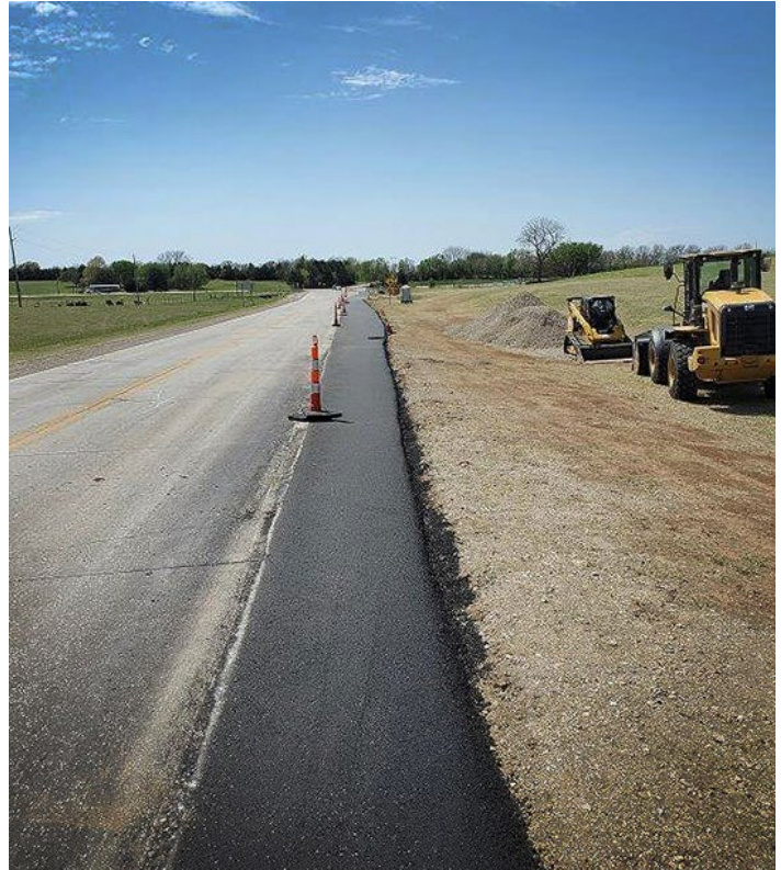
A view of some of the early work on the U.S. 166 project, at the west end, near the junction with U.S. 81. Photo by Therone Askins, District Five
