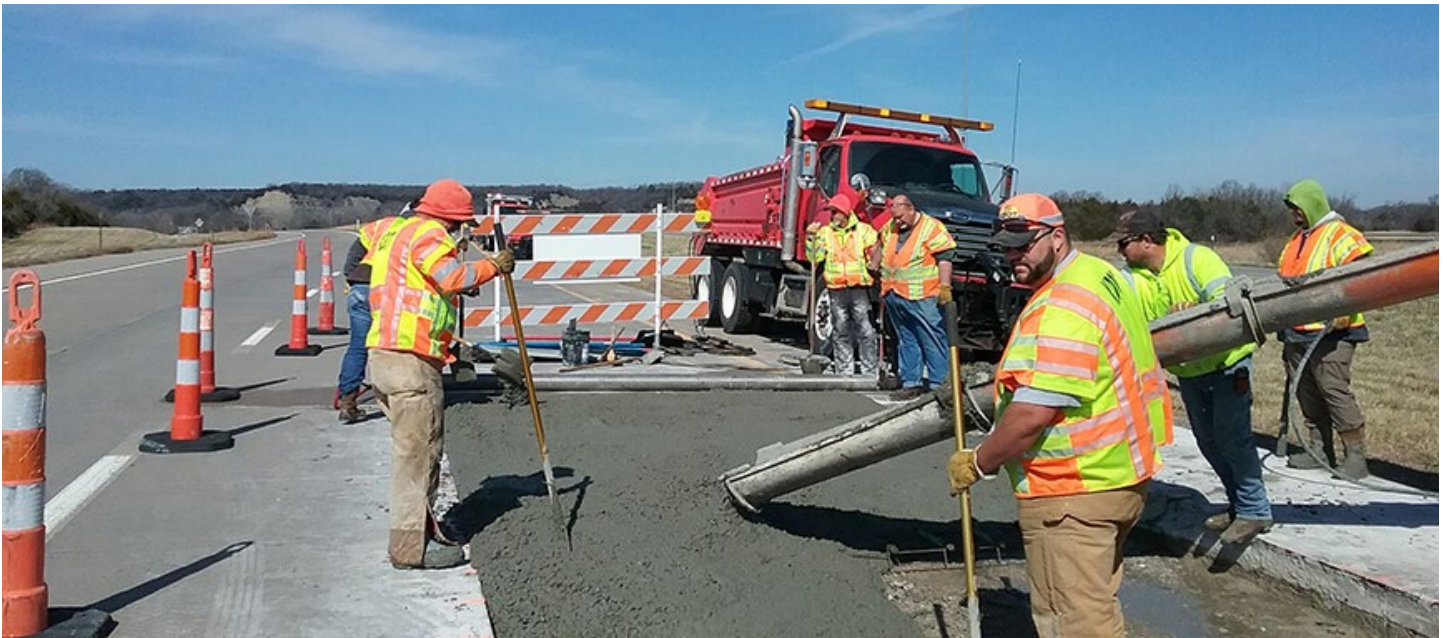
KDOT employees from the Independence office make full-depth concrete repairs on a section of U.S. 400 in mid-April. Photo by Priscilla Petersen, District Four
