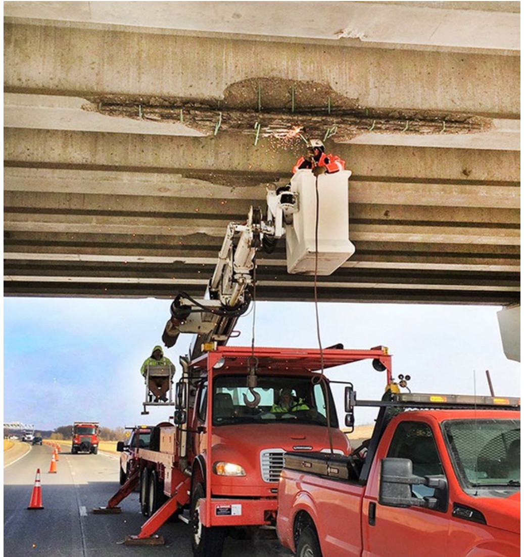
KDOT employees work together to make temporary repairs to a bridge hit by an excavator being hauled by a semi. Photo by Matt Mackeprang, District One
