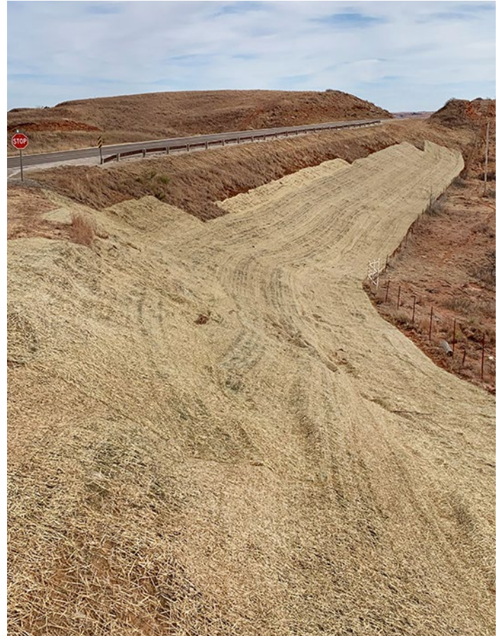
A cleared section along U.S. 160 in Barber County. The cleared area is covered with erosion-control blankets after it has been seeded. Photo By Scott Mullen
