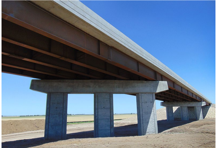
K-14 realignment progress continues - the new bridge at Avenue V that goes over the new K-14 at Sterling, in Rice County. Below, a view of the mainline looking south from Avenue V. Photos by Craig Schartz, District Five
