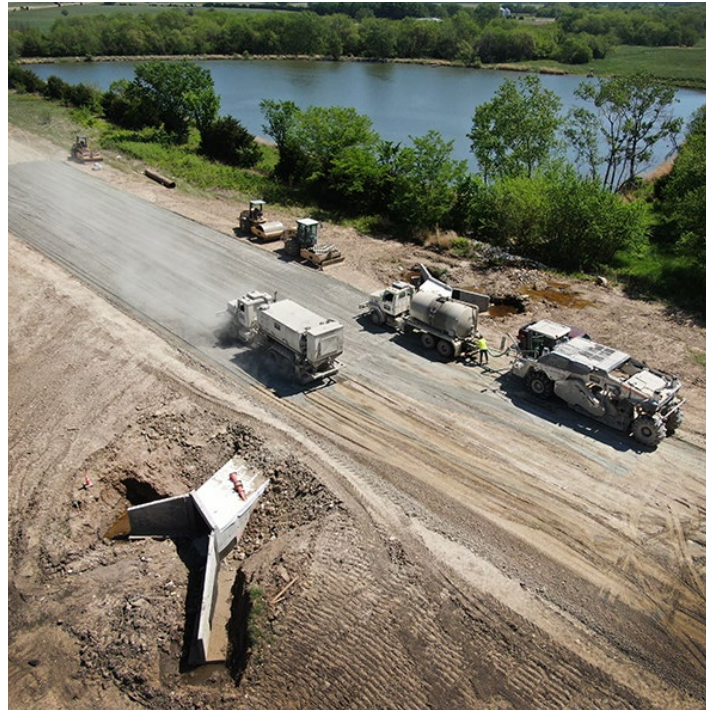
Rain has set back work on U.S. 169 in Neosho and Allen counties. Photo by Warren Ebberts, District Four
