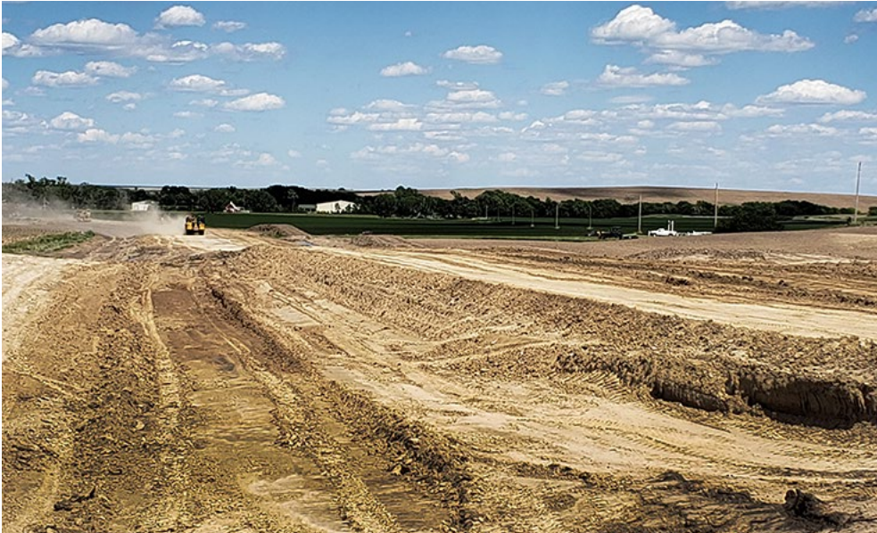
Grading and smoothing work proceeds on K-383 near Woodruff. Before Memorial Day the roadbed and entrances from 500 Road to the cemetery were smoothed out so people had access over Memorial Day weekend. Photo by Lisa Mussman, District Three.
