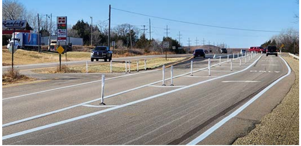
This photo shows changes made recently to westbound U.S. 24 at the K-13 intersection. Photo by Kate Craft, District One
