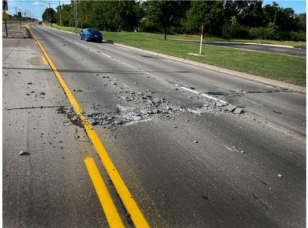
A blowup, since repaired, that occurred in June on U.S. 81 in Haysville. Photo by Mike Luna
