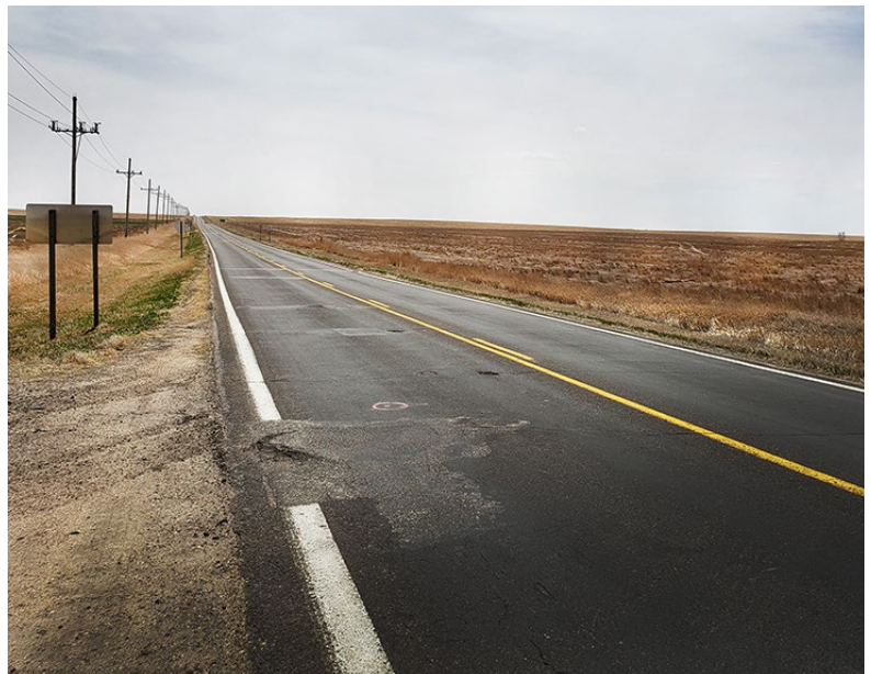
Looking south on K-123 near the K-383 junction in Decatur County. The reconstruction project will widen the pavement to 26 feet, including 1-foot asphalt shoulders. Photo by Lisa Mussman, District Three
