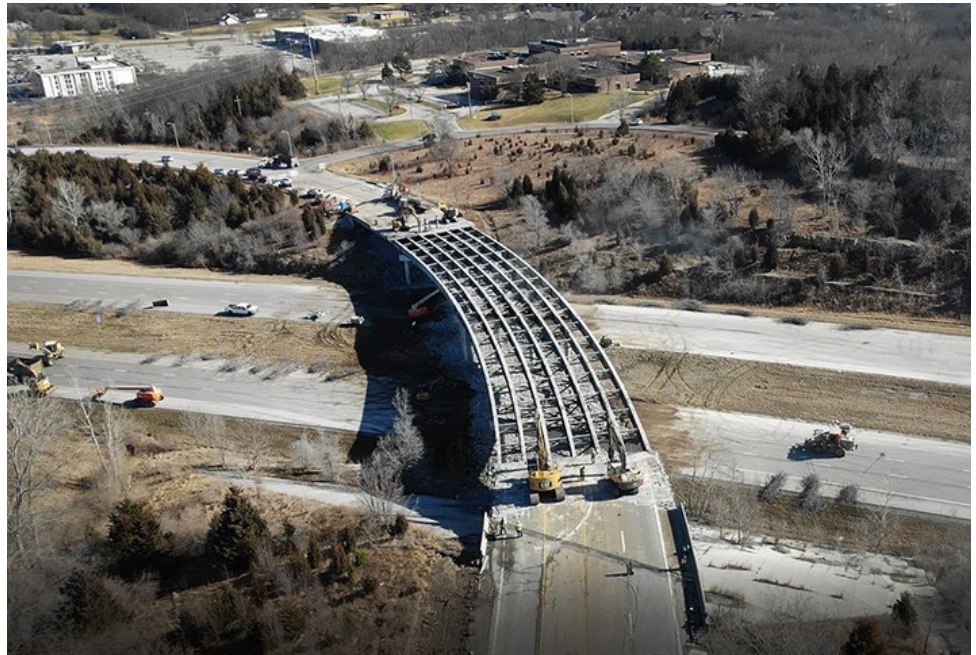
This aerial view of the Renner Road bridge demolition work in the Kansas City metro area shows a very uncommon occurrence - no traffic on I-435 below - just a few vehicles involved in the weekend project. Photo by Ian Stringham, District One.
