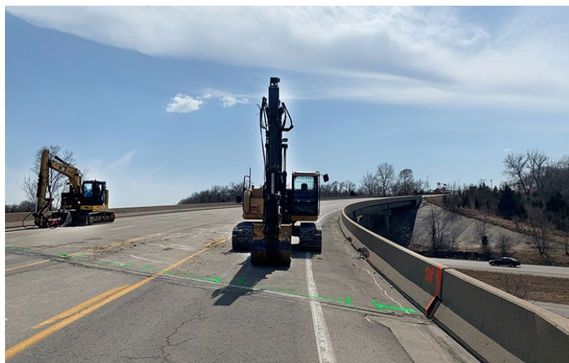
Equipment and markings were in place on the Renner Road bridge for preparation of the bridge deck demolition. Photo by Delaney Tholen, District One.
