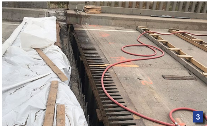
1/2. Recently, the crew broke up the concrete to remove the north end of the joint, then cleaned the joint on the U.S. 83 Business/South Main bridge project in Garden City. 3. The north half of the joint has been repaired, and the final concrete pour is scheduled soon. The bridge is expected to be re-opened by mid-September. Photos by Lisa Knoll, District Six
