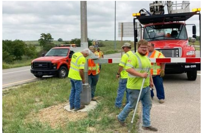
District Two employees work to install the new crossbar barricades. Photo by Vance Donahue, District Two
