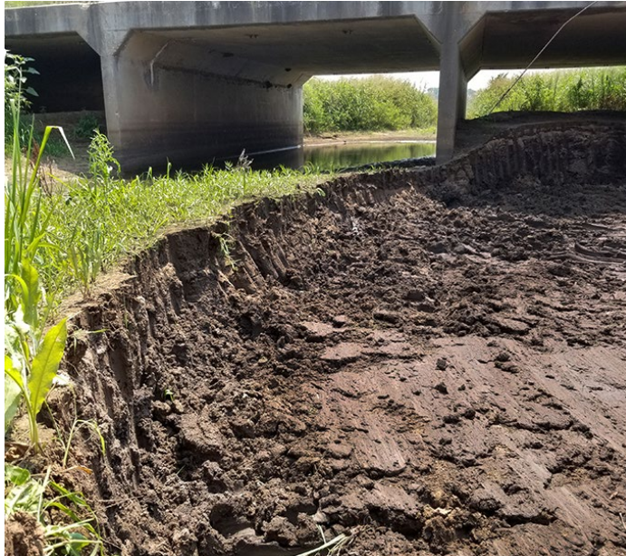
A view of the dirt removal earlier in the job (above) and a view once it was completed (below). Photos by Tim Potter and Marissa Martinez
