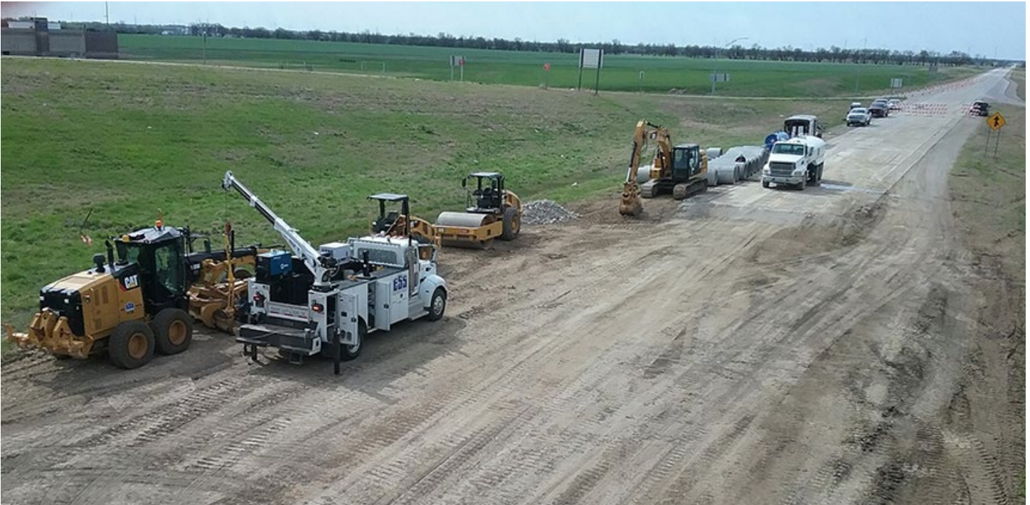
The U.S. 169 driving surface comes to an abrupt end at the 35th Street interchange at Chanute. A project to reconstruct U.S. 169 in Neosho and Allen counties began in March. (Photo by Priscilla Petersen, District Four)
