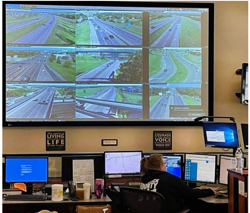
The WICHway Traffic Management Center now provides service 24 hours a day for the traveling public across Kansas. Photo provided
