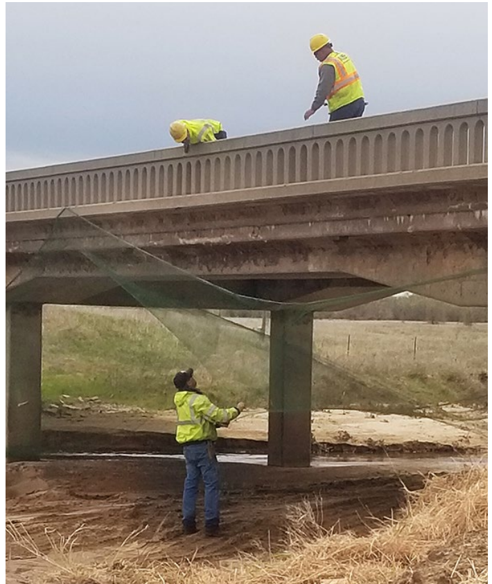
In the photos above and below, workers installed nets under the K-11 bridge over Goose Creek in Reno County on March 12. Photos by Jennifer Lee
