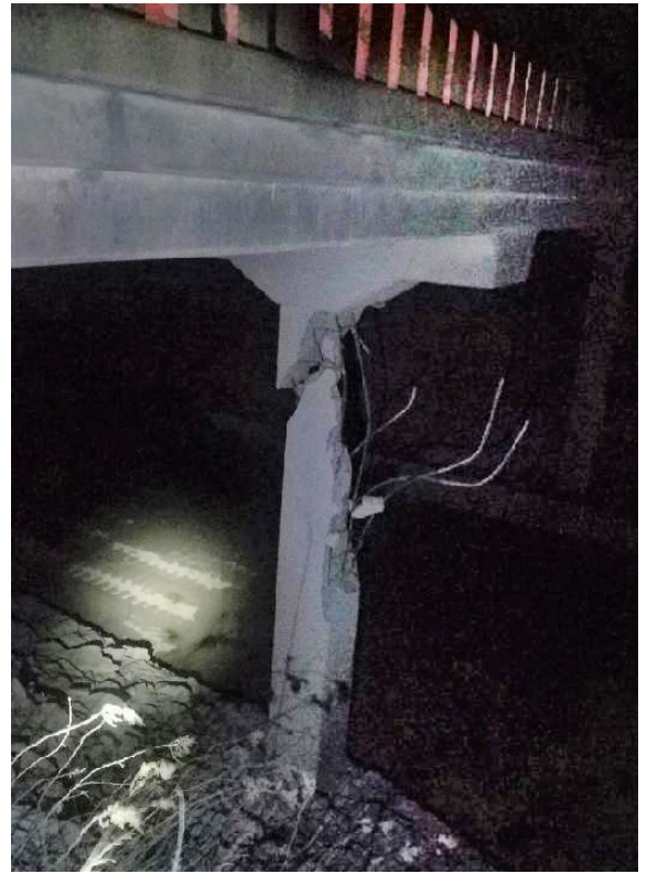
This bridge column underneath K-39 did not survive an encounter with an off-road dump truck. Photo by Wayne Nelson, District Four
