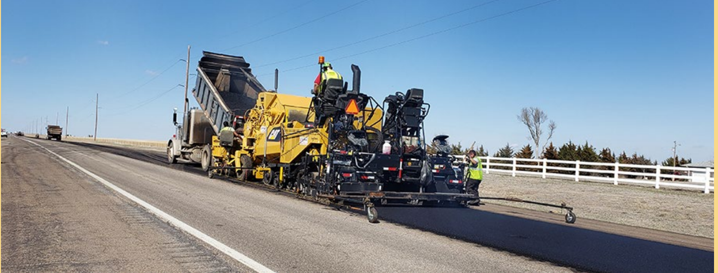
A mill and overlay project on U.S. 183 in Rush County was part of pavement preservation. Photo by Neisha Vetter, District Five
