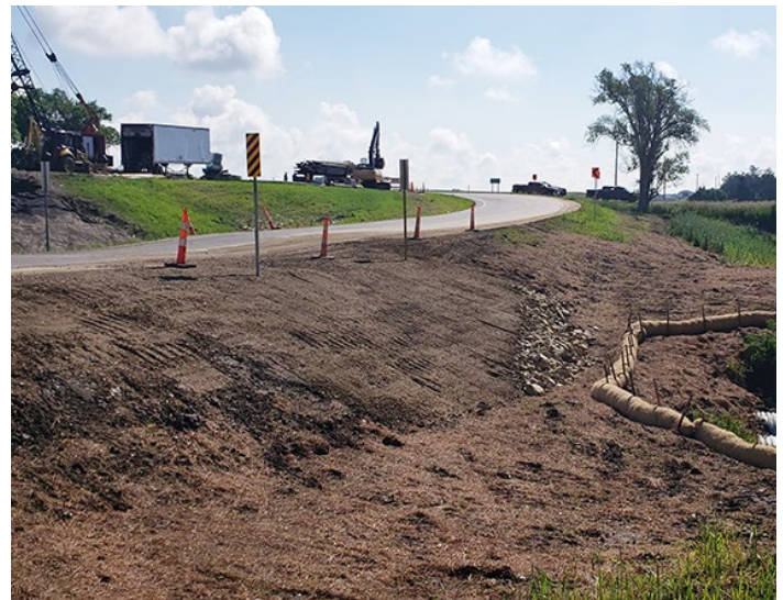
Crews from KDOT and Stone Sand Co. of Great Bend were able to quickly repair the damage with a mixture of stock granular and AS-1 materials. Photos by Hays Construction office and Penco Engineering
