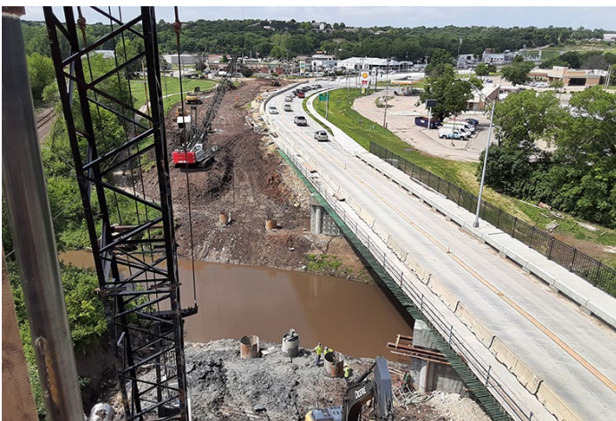
Construction on the K-18 bridge in Manhattan is in the final phase. Photos by Joe Haug, District One
