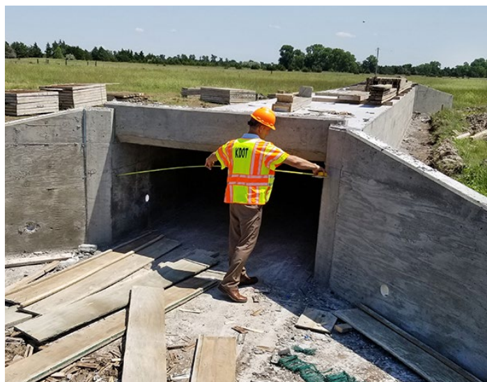
District Engineer Brent Terstriep measures a new box culvert during his tour of the K-14 project. Photo by Tim Potter
