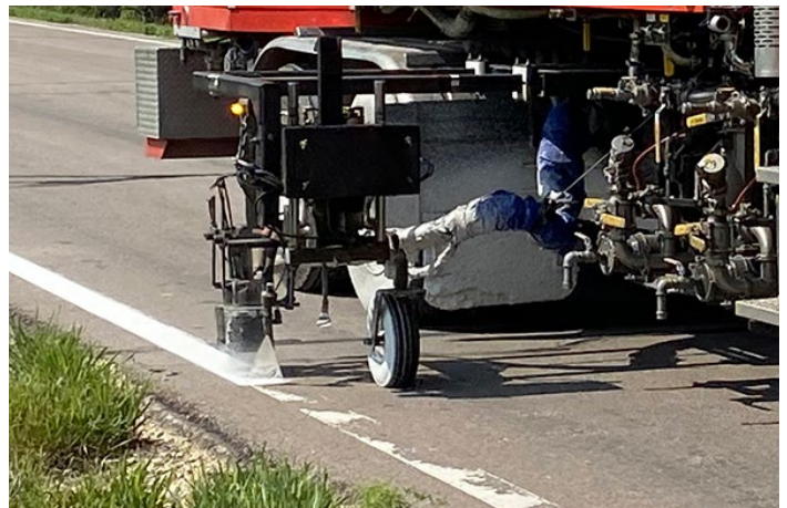
Paint and glass beads are applied to the roadway. Photos by Ashley Perez, District Two
