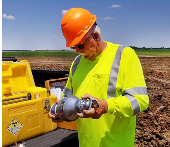
Engineering Technician Midpoint Rick Tomlinson shakes a Speedy as part of a soil density test on the K-14 realignment in Rice County. Below, other equipment he uses as part of the test: a ground probe and a set of scales. Photos by Tim Potter
