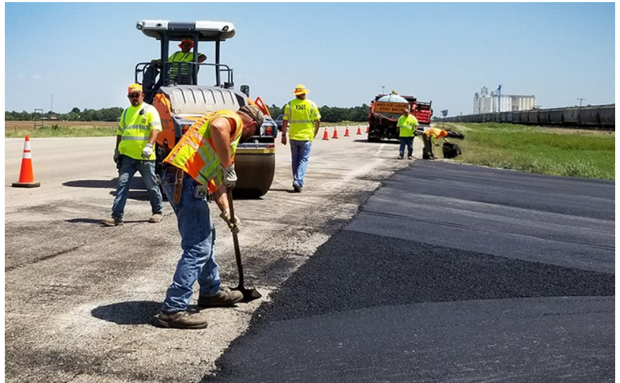
Above and below, a combined team of District Five crew members tackled an overlay job on U.S. 50 near Walton on an extra hot and humid day. Photos by Tim Potter, District Five
