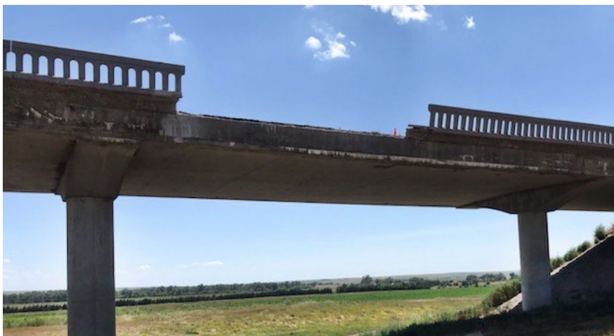
In the photos above, crews recently removed a portion of deteriorated rail as part of the emergency repairs currently underway on the bridge. Photos by Wildcat Construction
