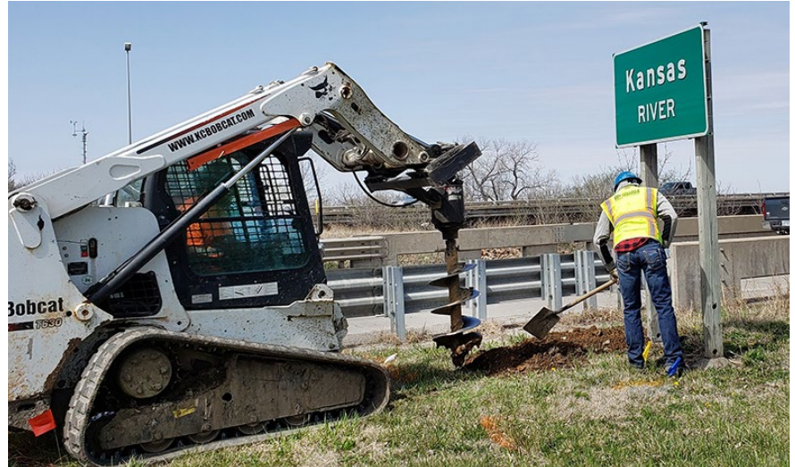
A contractor's employee works on a post hole for a new sign installation. Photos by Bill Bartron, Headquarters
