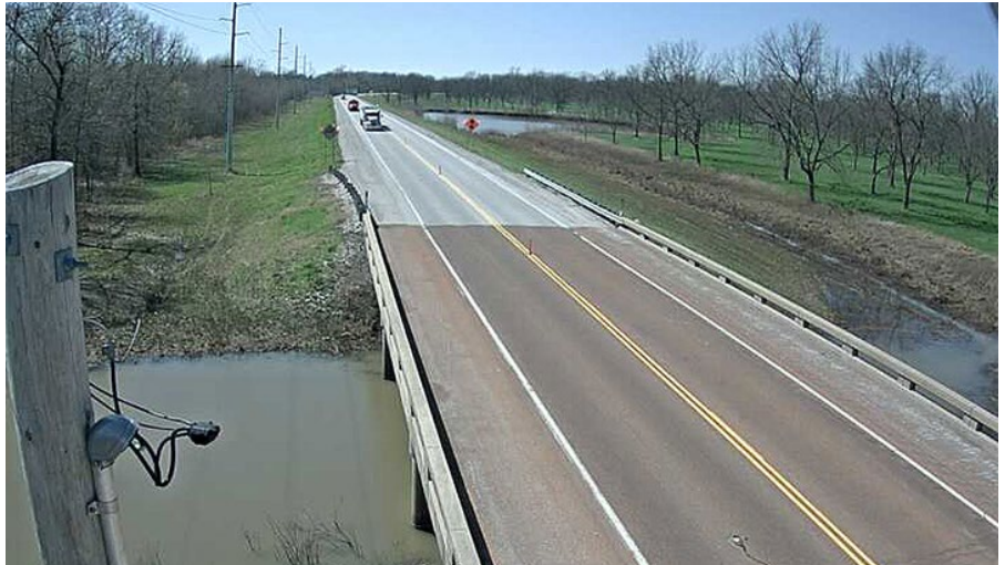
A KanDrive camera captures an aerial view of a section of the marshy construction zone where six bridges are being replaced on U.S. 166.
