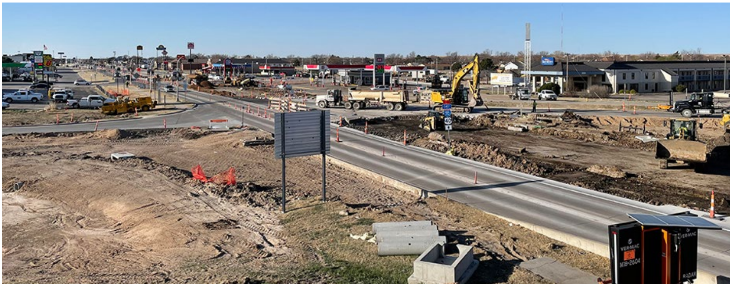
Realignment work on the I-70 ramps in Hays continues. Photo by Bill Koerner, Kirkham-Michael
