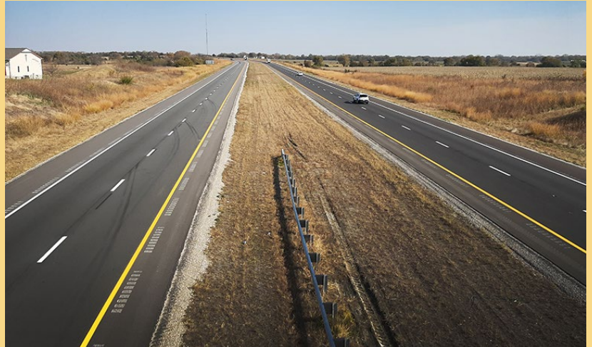
Work on a major I-35 resurfacing project was completed this autumn. A one-inch reflective crack interlayer with a three-inch asphalt overlay was placed on I-35 between mile markers 179-191 in Franklin County. The resurfacing replaced failing pavement on this section. Bettis Asphalt & Construction was awarded the $12.4 million construction contract. Steve Rockers' road squad designed the project. Photo by Donna Schmit, District Four
