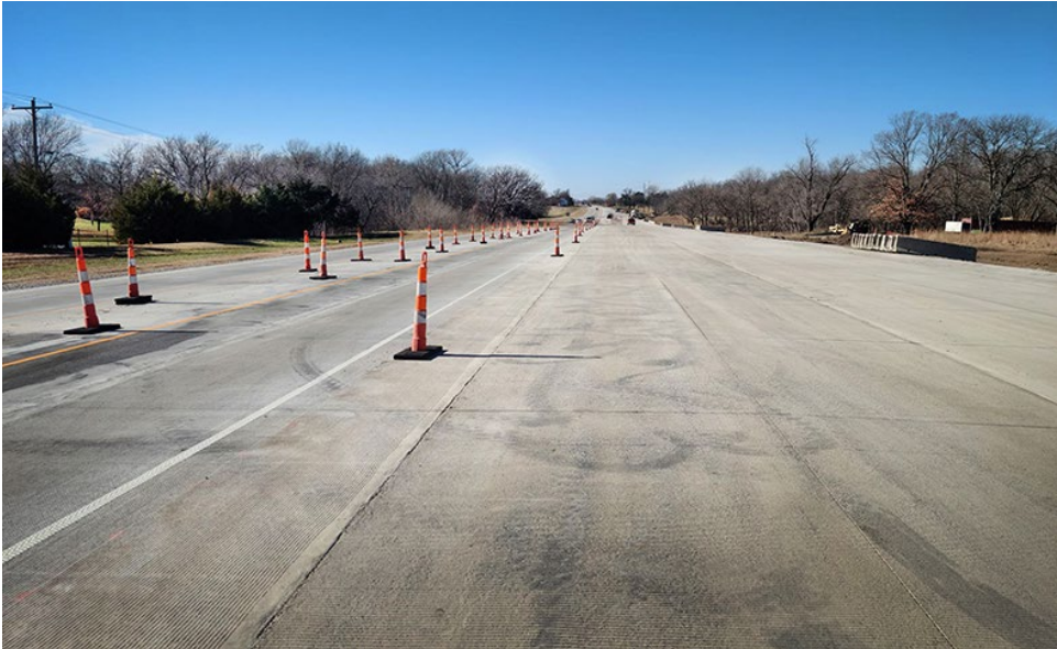
Work is wrapping up on U.S. 50 in Lyon County. Photo by Dustin Hardin, District One
