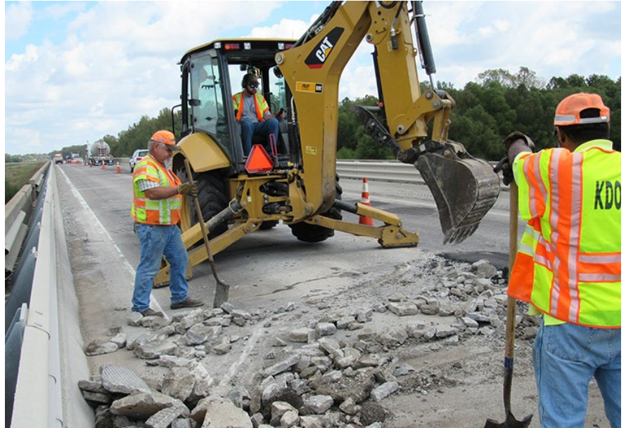
In the photos above and below, KDOT crews patch and place an asphalt overlay on the U.S. 59 bridge over the Neosho River. Photos by Joe Engle, District Four
