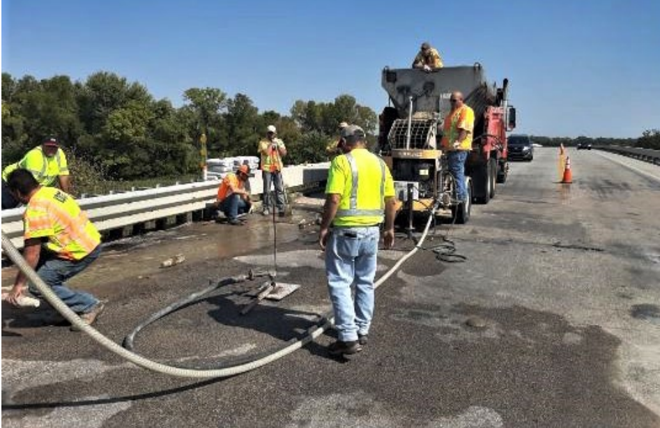
Crews from districts Four and Five perform mudjacking on a bridge approach along K-47 west of St. Paul. Photo by Wayne Nelson, District Four
