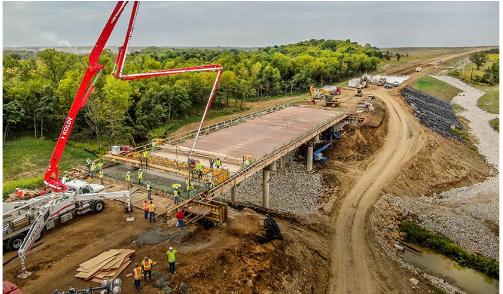
Warren Ebberts took the aerial photo of U.S. 169 reconstruction in Anderson County above while Rowdy Glaser took the aerial photo below.
