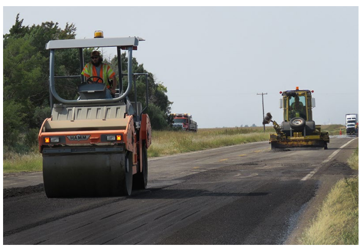
Above and at right, Burke Koehn and Jamie Davis from the Scott City Subarea overlay asphalt on K-96 in Scott City.
