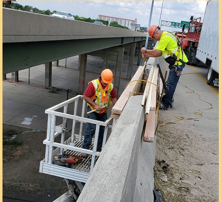
Bridge Crew Supervisor Darren Bailey, in the derrick truck basket, and Craig Kenyon, Bridge Crew Equipment Operator Senior, repair barrier wall on U.S. 54 in Wichita. Photo by Dustin Covert, District Five
