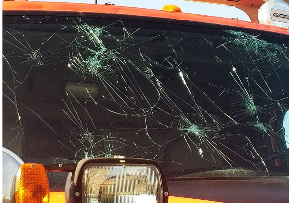
Above , hail shattered a KDOT vehicle’s windshield at the Mankato Subarea office during an Aug. 14 storm. Below left , several windows were broken on the Subarea office. Below right , the computer near the window was soaked and had broken glass. Photos by Doug Newquist, District Two
