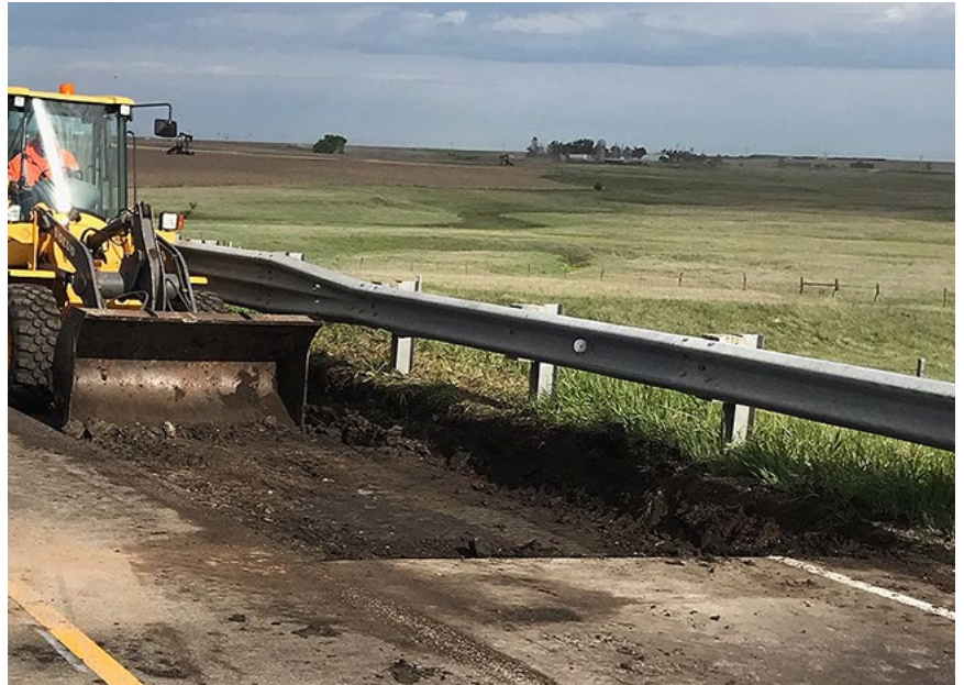
KDOT crews quickly repair a pothole that formed in an I-70 work zone. Photo by Max Dirks, District Three
