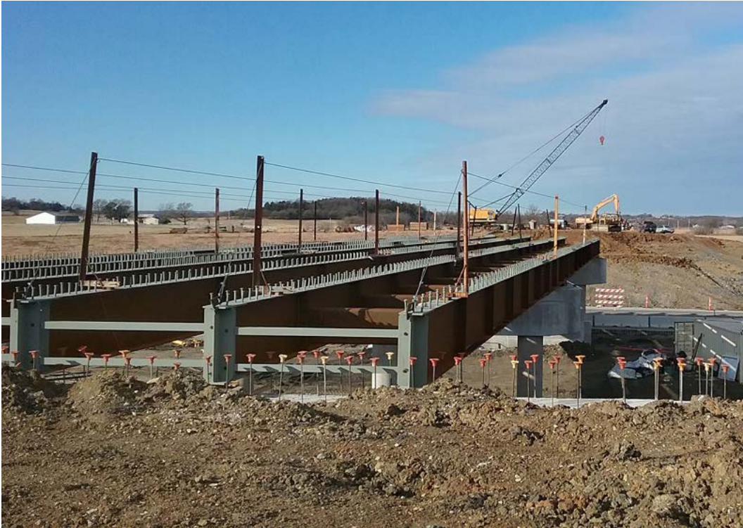
Work continues to progress during the winter months on the interchange construction at U.S. 169 and U.S. 160 junction in Montgomery County. The new bridge above U.S. 169 is taking shape, and reconstruction has started on the access road east of U.S. 169. Kings Construction Company is the primary contractor on the $12 million T-Works project, which KDOT expects to open to traffic this summer. Brad Rognlie's bridge squad and Stephen Bass/Greg Gonzales' road squads designed the project.
