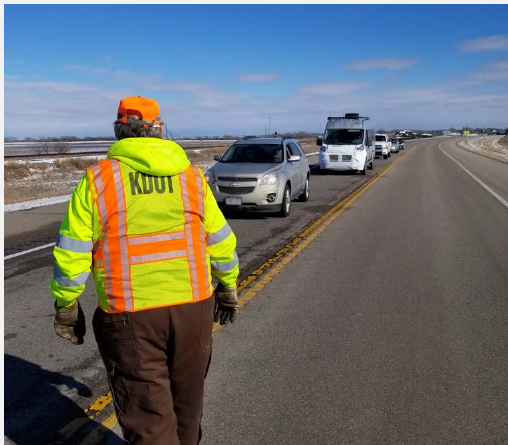
Numerous KDOT employees assisted in the efforts to stop and reroute traffic around the closure on U.S. 54 west of Pratt. Photo by Tim Potter, District Five
