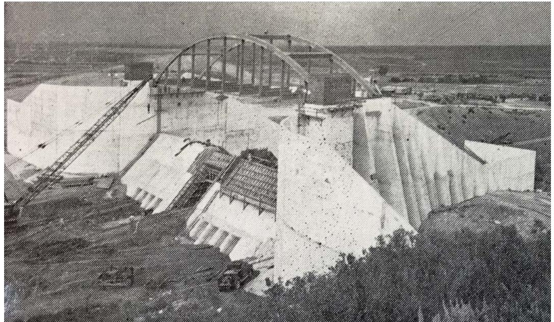
A historical photo shows the final truss being hoisted into place on K-147. Records indicate that it took part of only three working days to erect the steel trusses.
