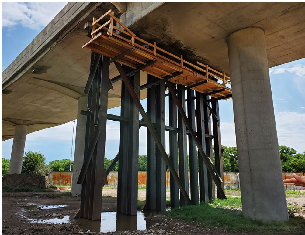
Steel falsework holds up the box bridge on I-135. The bridge was lifted one-fourth inch while new bearings are installed. Photo by Tracy Crockett
