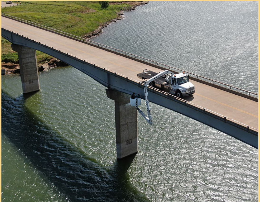
Observation of the inspection work on Hell Creek Bridge over Wilson Lake took place recently with Lynn Berges, Local Bridge Engineer, serving as UAS pilot and Karlton Place as visual observer. Photo by Lynn Berges, Headquarters
