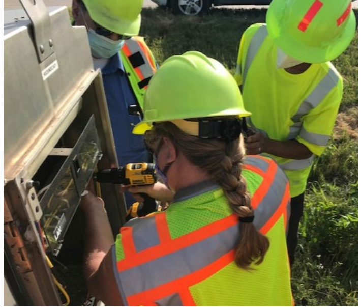
KC Scout technicians install new communication equipment in the cabinet. Photos provided by KC Scout
