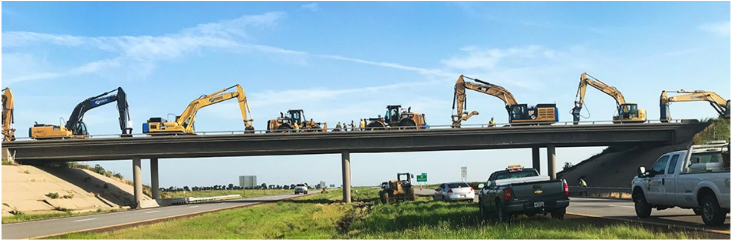
Workers make preparations for the Avenue A bridge to be demolished. Photo by Joe Palic, District Two
