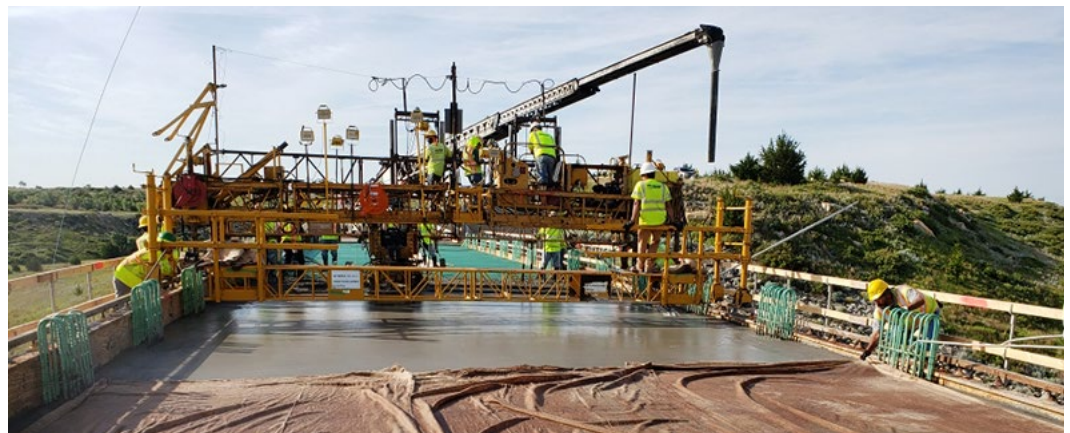
Crew members from Wildcat Construction pour the new bridge deck on July 23. The bridge is expected to be reopened to the traveling public in mid-August. Photos by Wildcat Construction and Lisa Mussman, District Three
