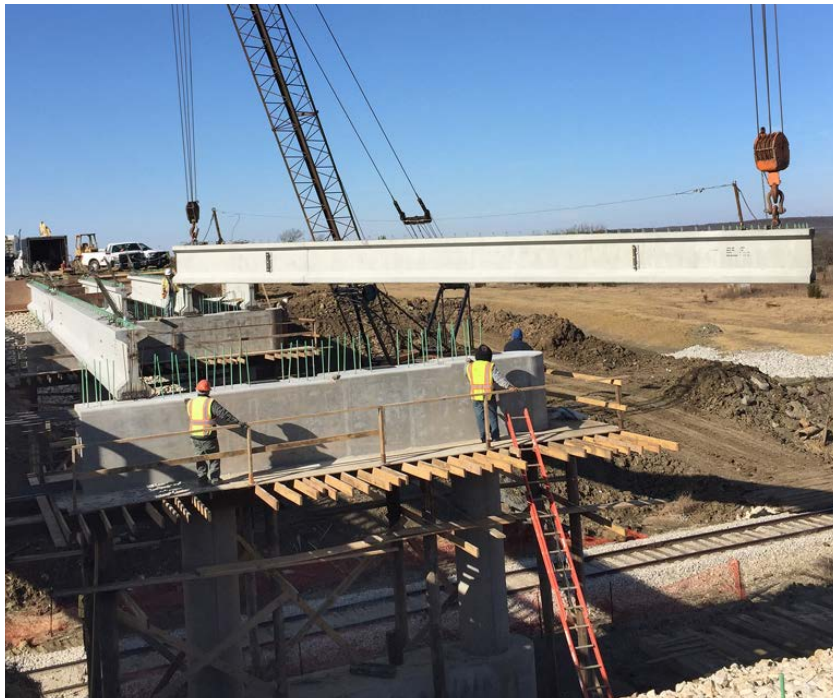
Construction continues on the new South Kansas & Oklahoma Railroad overpass at the U.S. 166/U.S. 75 junction.
