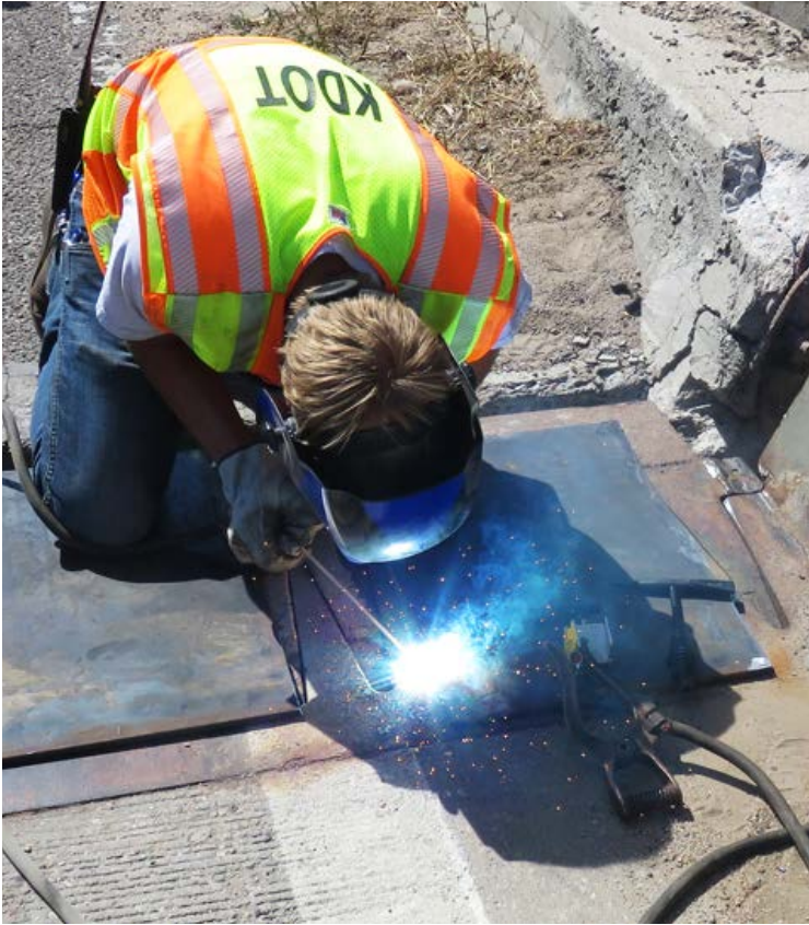
Landon Baier, Equipment Operator from the District Six Bridge Crew, welds metal plates in place on the U.S. 83 bridge south of Garden City.
