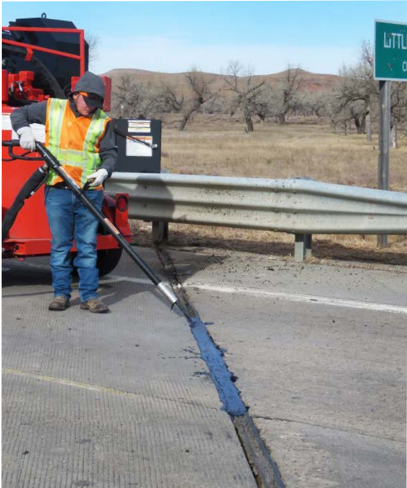
Kyle Hughes, Equipment Operator at the Ashland Subarea, repairs the expansion joint on the U.S. 160 bridge over Little Sandy Creek in Clark County.
