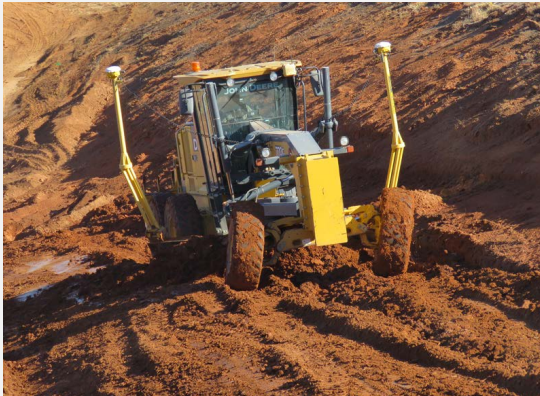
Stoppel Dirt, LLC of Sublette recently completed a grading and dirt work project on U.S. 160 in Clark County.
