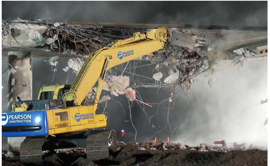
A 1960s era bridge was demolished over I-235 in north Wichita earlier this summer.
