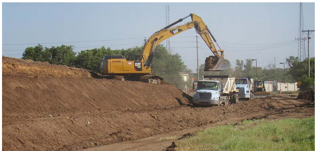
To construct new ramps at the I-235/Broadway interchange, dirt had to be removed.
