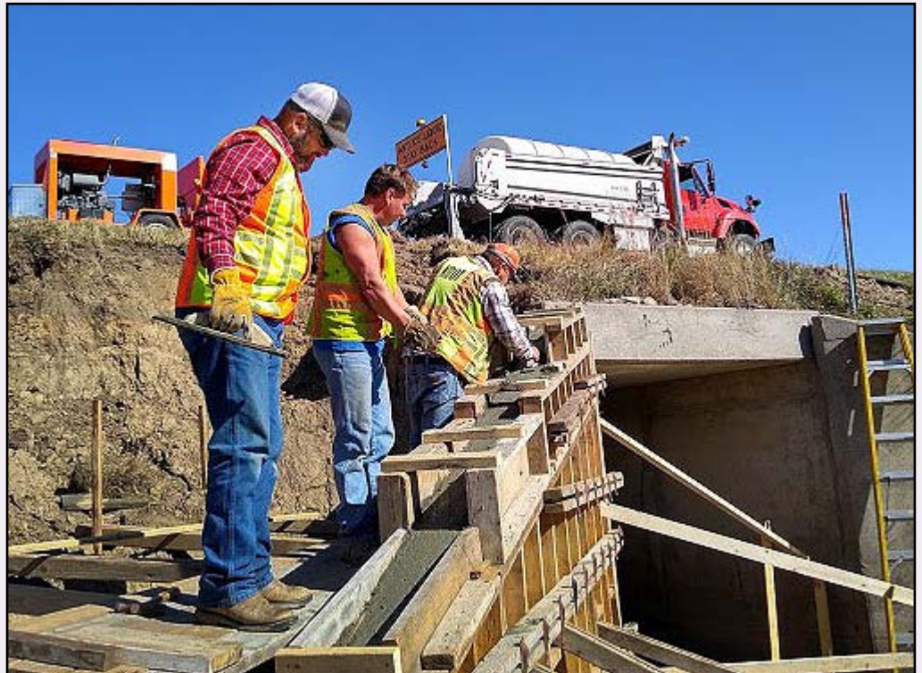
From left to right, David Casper, Highway Maintenance Supervisor in Concordia, Donnie Burkholder, Equipment Operator Senior on the District Specials Crew in Salina, and Jason May, Area Supervisor in Marion, work together to make quick repairs on a culvert on U.S. 24 near Beloit. Photo by Doug Newquist, District Two
