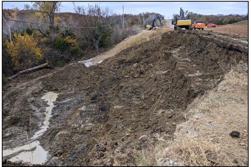
Stair-stepping 'benches' are formed at the slide as dirt is removed. Photo by Denny Martin
