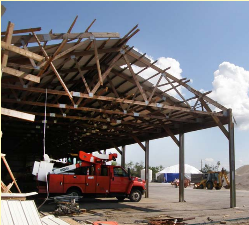
An EF-3 tornado moved through the city of Eureka last spring and damaged homes and buildings at the KDOT subarea office.
