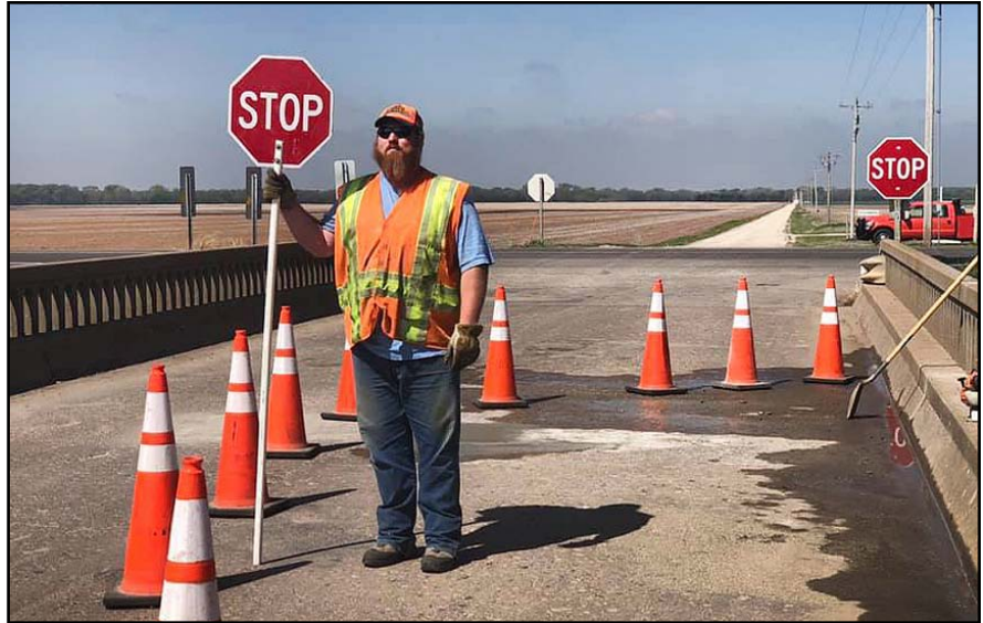
Rocky Lindgren, Equipment Operator Senior from Salina, flags traffic in a work zone.
