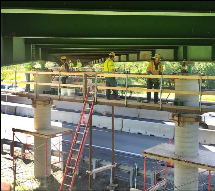
Above, crews raise the vertical clearance of a bridge located at mile marker 102 on I-35/KTA. Photo by KTA
