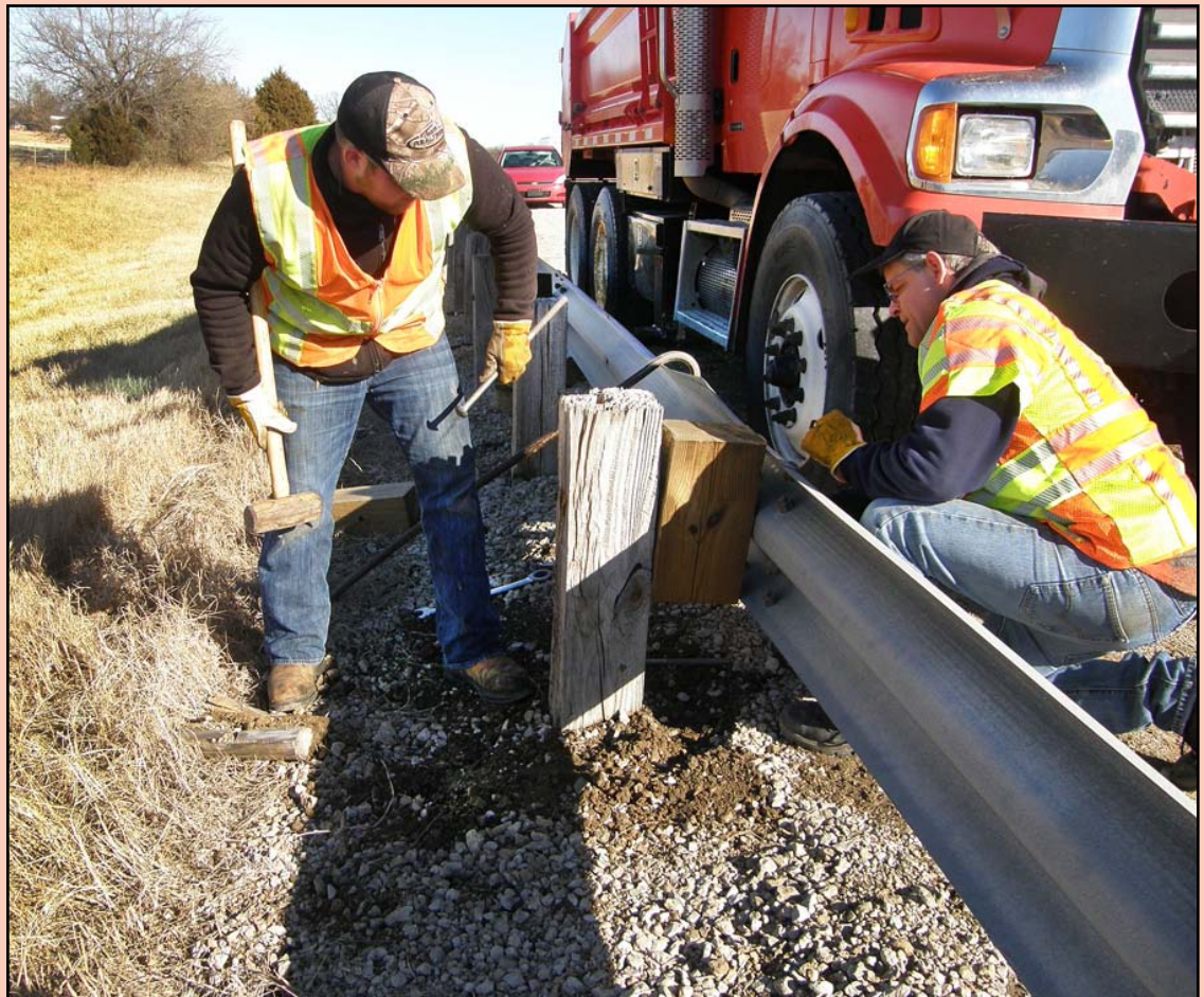
Andrew Snider and James Hasselbring, Equipment Operators at the Independence KDOT office, make repairs to a guardrail post that was damaged during a recent crash on U.S. 166. Maintenance activities along the highways are continuing during the milder days of winter.
