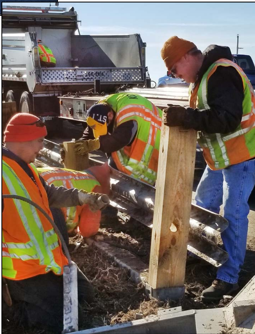
From left to right, KDOT employees Rocky Lindgren, Tim Frederiksen, Terry Shank and Ben Workman repair guard rail along I-135.
