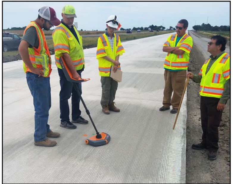
The National Concrete Pavement Technology Center team members demonstrate non-destructive thickness determination of concrete pavement on I-70 in Gove County. Instead of cutting a pavement core to determine thickness, a pad is placed on the base or subgrade. After the concrete pavement is placed, the pad is relocated and the pavement thickness is determined by rolling the instrument on the new pavement above where the pad was placed. Photo by Rob Percival, District Three
