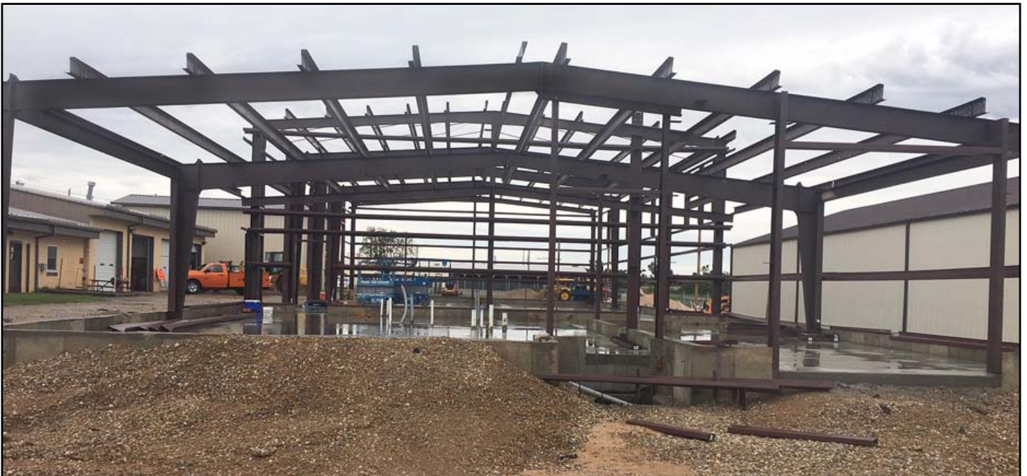
Construction is underway on the new office of the KDOT Subarea in Eureka. An EF-3 tornado touched down in Eureka in late June 2018. The existing office, left, and other subarea buildings received extensive damage. Photo by Jeff Marks, District Four
