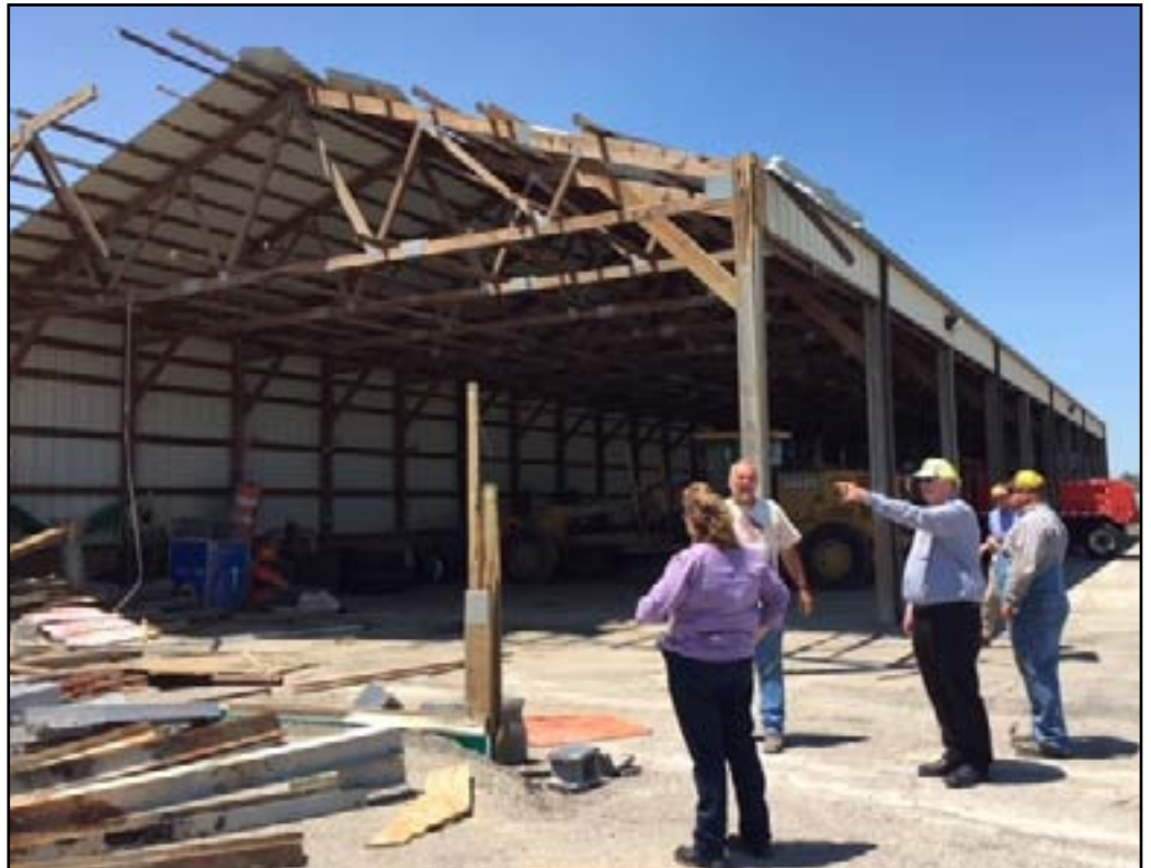
At left, State Transportation Engineer Catherine Patrick and Director of Operations Larry Thompson, center, survey tornado damage of the cold storage building at the Eureka shop.
